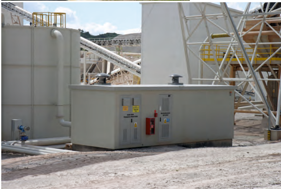
Forced ventilation, system with filters
