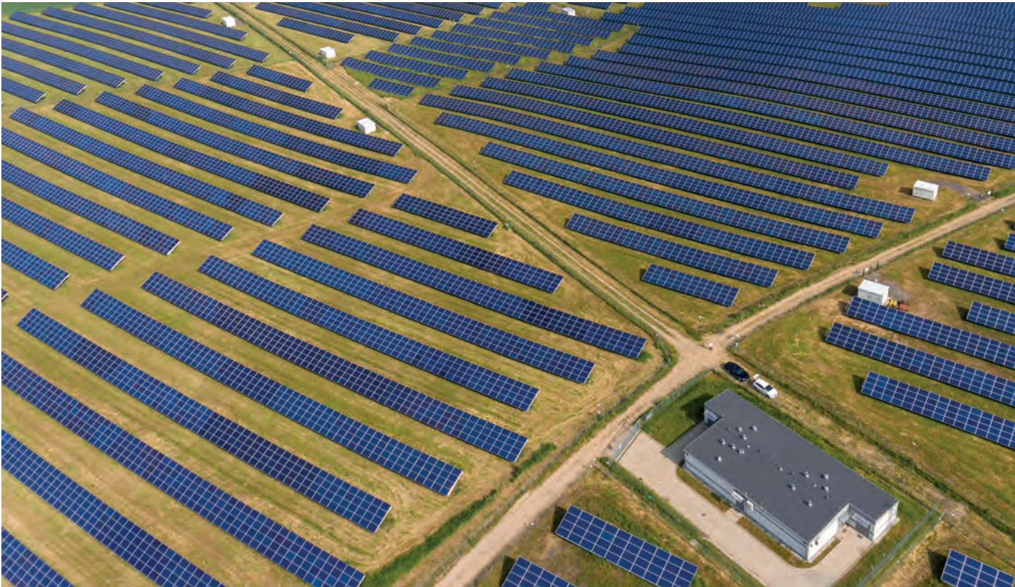
72 stations with a capacity of 1 MW equipped with MV and LV switchgears produced by ZPUE S.A.
