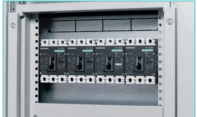
Outgoing feeders set with SENTRON 3VL circuit breakers
